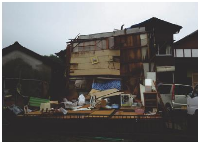
DI 1: Wooden residential houses or stores DOD 8: Major destruction/collapse of main structures frames (LB 55m/s) (Chikugo City, 28 September, 2016)
