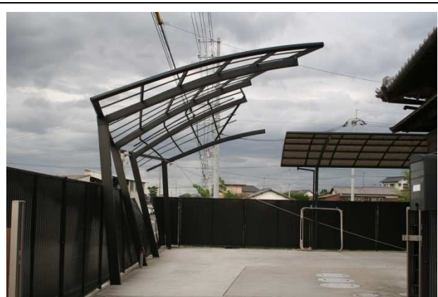
DOD = 2 Wind-related inclination of frames (Application of UB to a three-column cantilevered carport without walls) Courtesy of Institute of Technology and Science, Tokushima University
