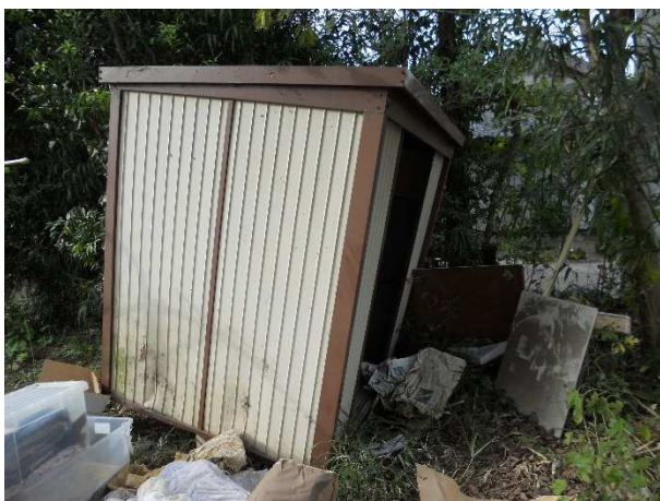
DOD = 1 Slippage/overturning with content of 0 – 300 kg
