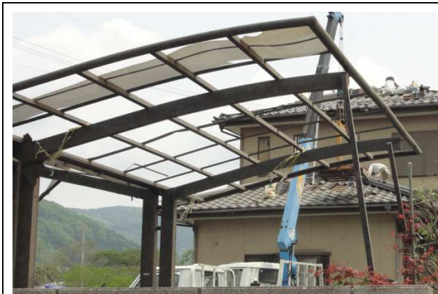
DOD = 1 Debris-related destruction of roofing panels Courtesy of Wind Engineering Research Center, Tokyo Polytechnic University
