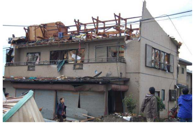
DOD = 7 Destruction/detachment of roof frames/components Courtesy of NILIM, BRI
