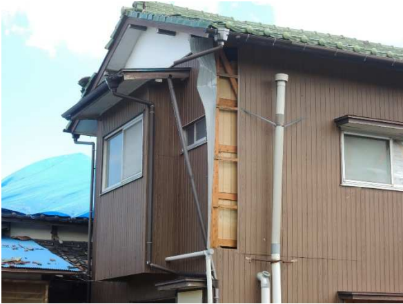
DOD = 6 Loss of metal wall cladding (Example of LB adoption due to a lack of connection resistance against pull-out force in surrounding damaged sections) Courtesy of NILIM, BRI
