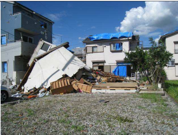
DOD = 8 Major destruction/collapse of main structures and frames (Example of LB adoption because the house was built before 1981.) Courtesy of NILIM, BRI
