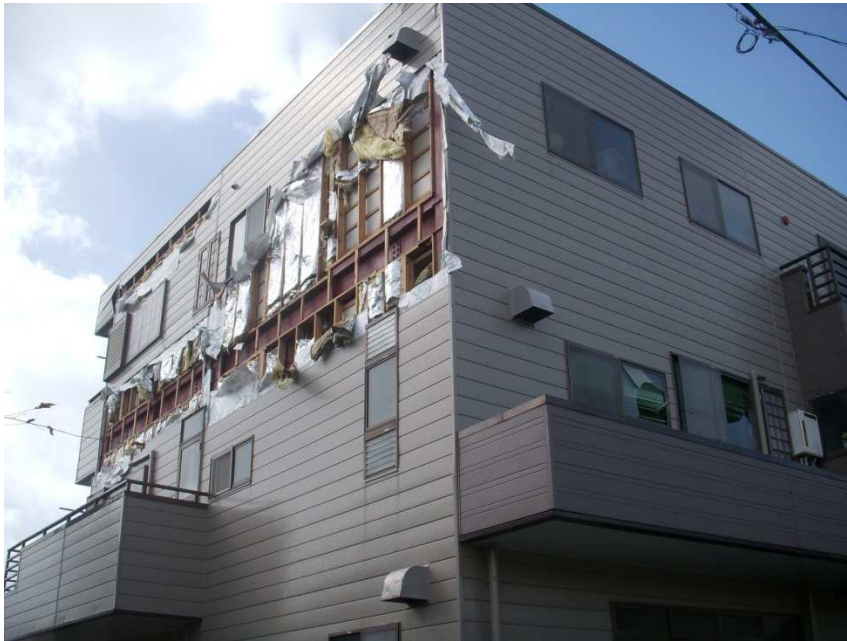
DOD = 5: Destruction/detachment of the eaves or the sheathing roof boards, deformation/loss of wall cladding Courtesy of Building Research Institute (BRI)
